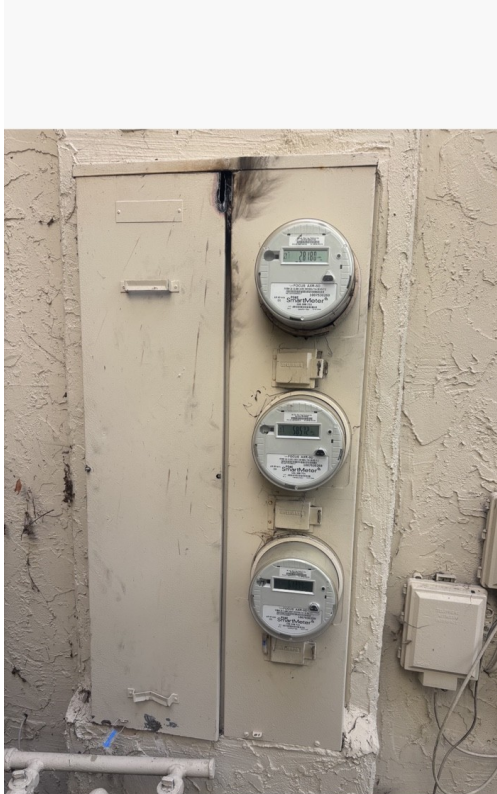
Arcing and heat damage at the upper cabinet seam
